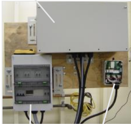
Circuit Control Panel
